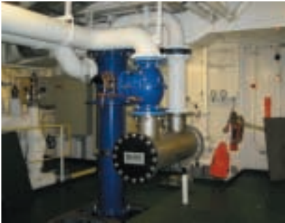
OptiMarin's OPTIMAR Ballast treatment System – based on solid separation and ultra violet irradiation – installed aboard the Regal Princess
